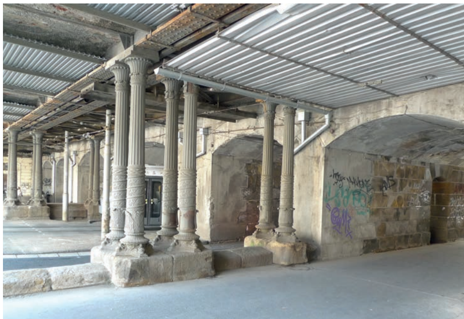
Brno, kamenný viadukt vedl v roce 1848 kusé koleje do výtopy Severní státní dráhy přes ulici Křenová, v roce 1869 rozšířen mostem na litinových sloupech. Foto Alena Borovcová, 2013. • Brno, in 1848 a stone viaduct was built to span Křenová (formerly Kröna) St.; it was used by a dead-end line of the Northern State Railway and led to the engine-house. In 1869 the crossing was extended when a bridge with cast iron pillars was built. Photograph by Alena Borovcová, 2013.
