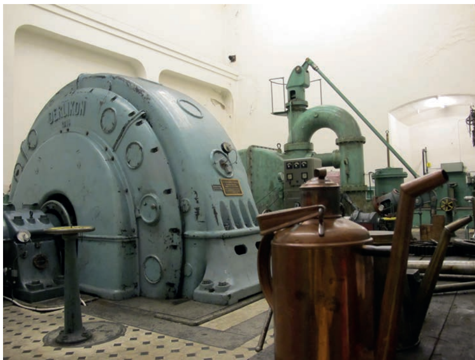
Rjukan, Sâheim Power Plant, the underground turbine generator hall above Sâheim. Photograph by Trond Taugbøl. • Rjukan, elektrárna Sâheim, podzemní strojovna. Photo Trond Taugbøl.
